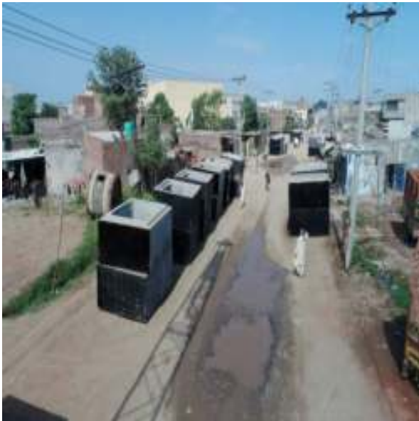
Picture 76: Single Cell Conduits laying is in progress near Sublime Chowk Site 1 Marala Road Sialkot
